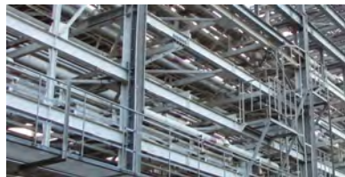
Overhead piping Reduces the risk of soil contamination (no buried piping)
