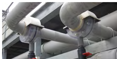
Double piping joints Monitoring and prevention of liquid leakages
