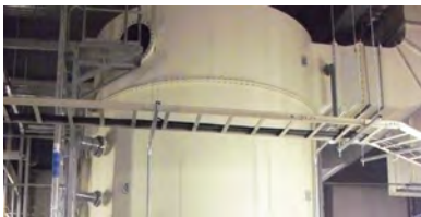
Waste gas scrubber Structures and specifications aimed at ensuring stable processing
